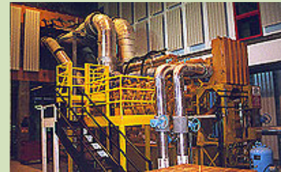
Image: Point Loma Wastewater Treatment 38
